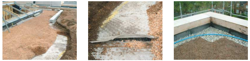
Above: Construction pictures of a green roof terrace at Moorgate Crofts Business Centre, Rotherham. Concrete blocks delineate the paved areas, with crushed brick beneath for drainage. The crushed brick and substrate sits on top of a filter mat, which lies on the plastic drainage layer (close-up picture). Further drainage is installed at the periphery, with pebbles also helping to protect the roof edge against wind eddies.
